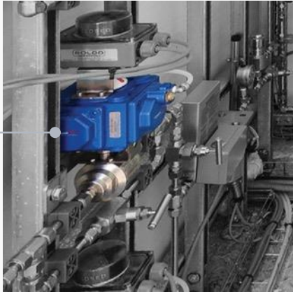
Hydrogen refueling station
